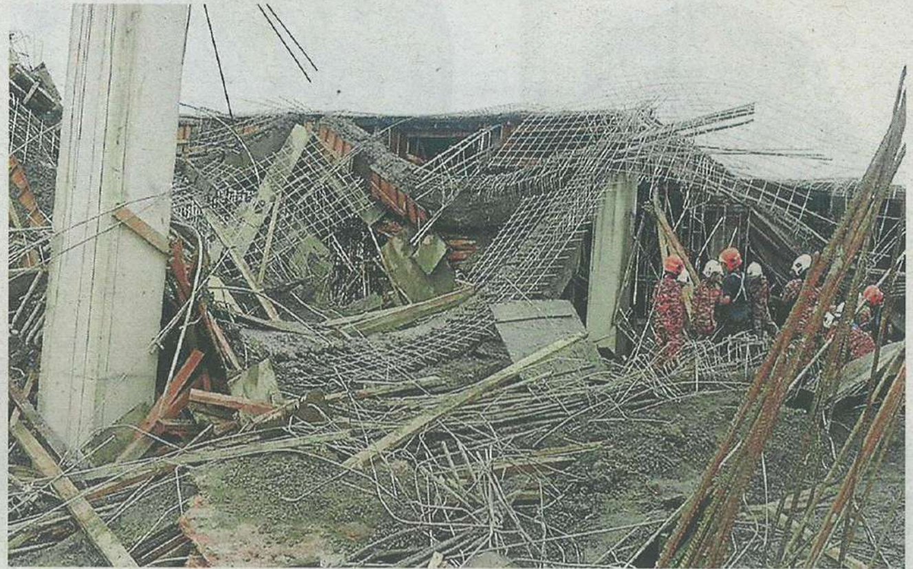
Deadly development: Fire Department personnel inspecting the scene of the deadly collapse in Ulu Tiram, Johor.
