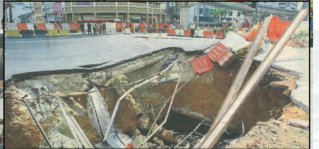
rush hour chaos: One of the two sinkholes that appeared at the Jalan Pudu-Jalan Imbi intersection yesterday, disrupting traffic flow. - Photo by MUHAMMAD SHAHRIL The day the earth moved Ongoing construction work on part of the Pudu Underpass project has caused the road above the tunnel to collapse leaving large holes at the intersection. 283
