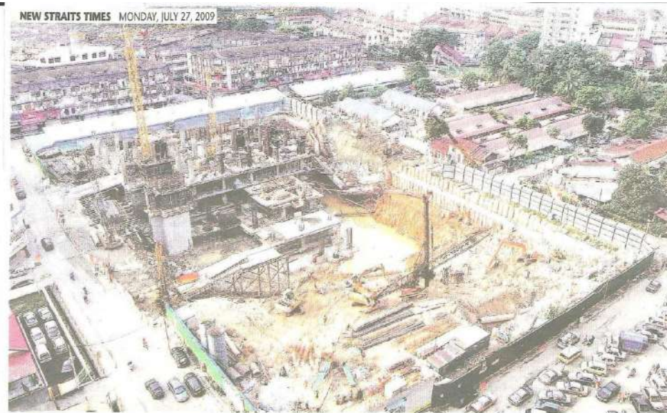
There is development on one side of the Lorong Gelugor cave-in, which occurred near the houses with blue roofs. — NST pictures by Ahmad Irfam Mohd Noor
