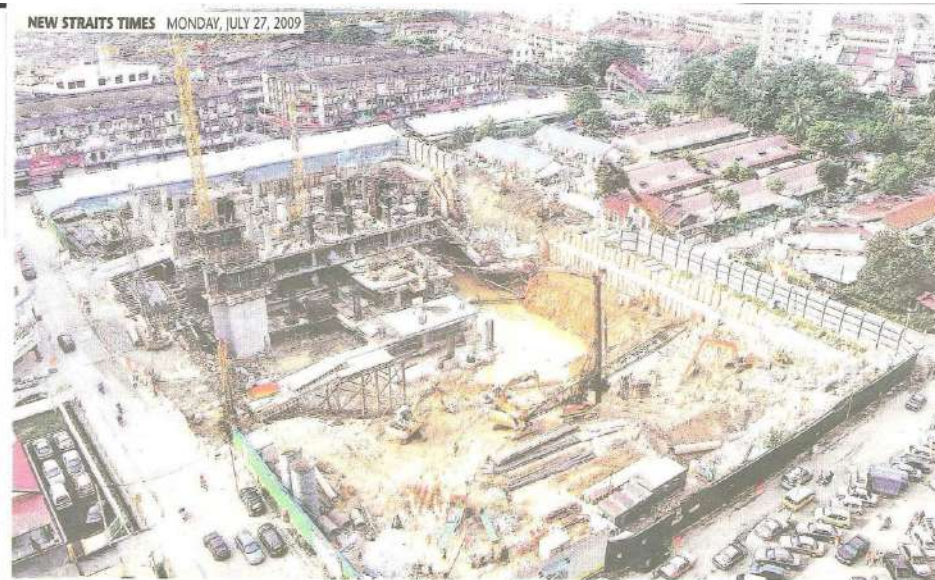
There is development on one side of the Lorong Gelugor cave-in, which occurred near the houses with blue roofs. — NST pictures by Ahmad Irfam Mohd Noor
