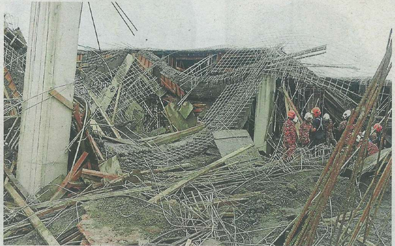
Deadly development: Fire Department personnel inspecting the scene of the deadly collapse in Ulu Tiram, Johor.
