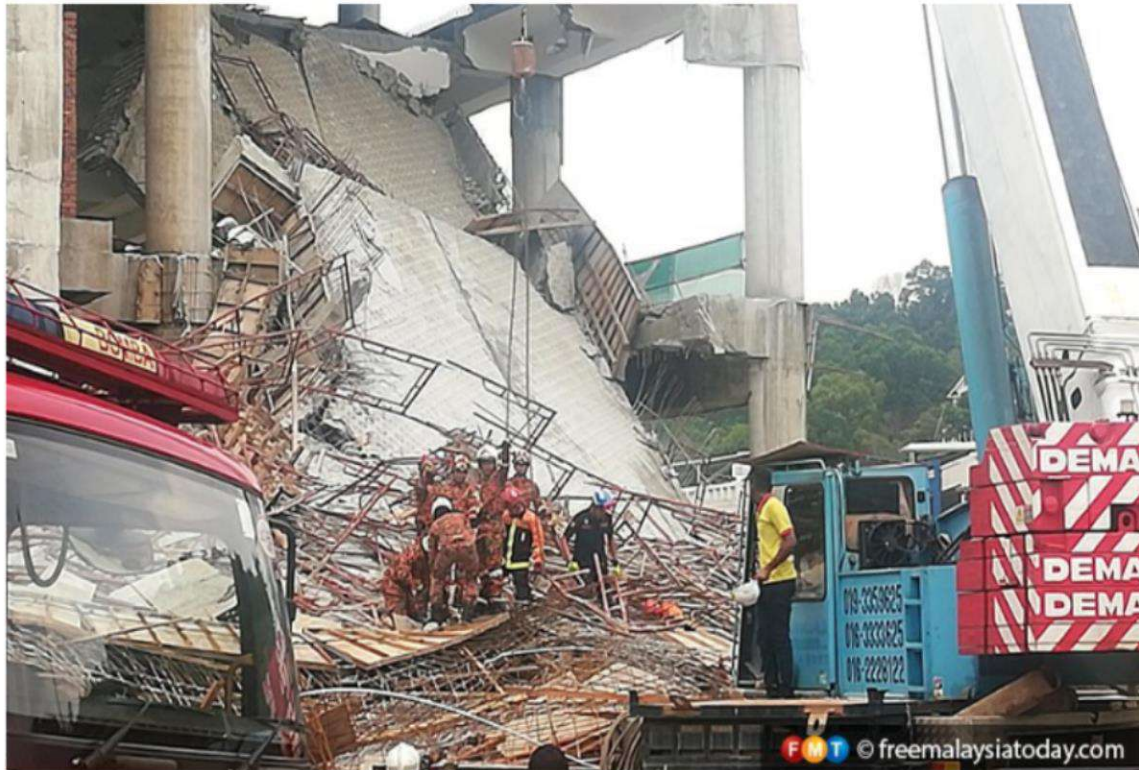
An Indonesian couple, working as construction workers, were killed when a building collapsed near the Gombak LRT station on May 23.
